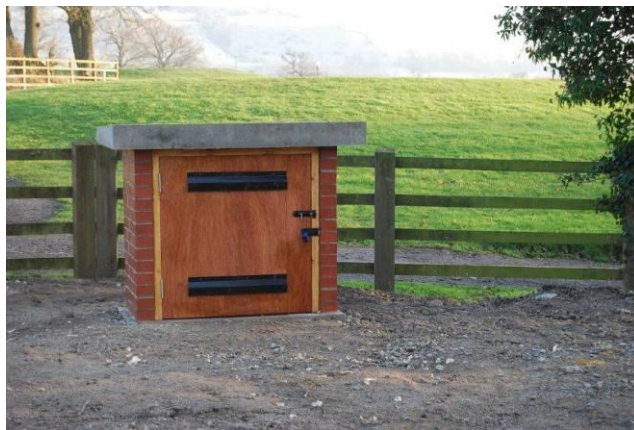
New meter house in car park
